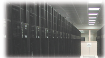
A large HPC datacenter (CEA-DAM)
